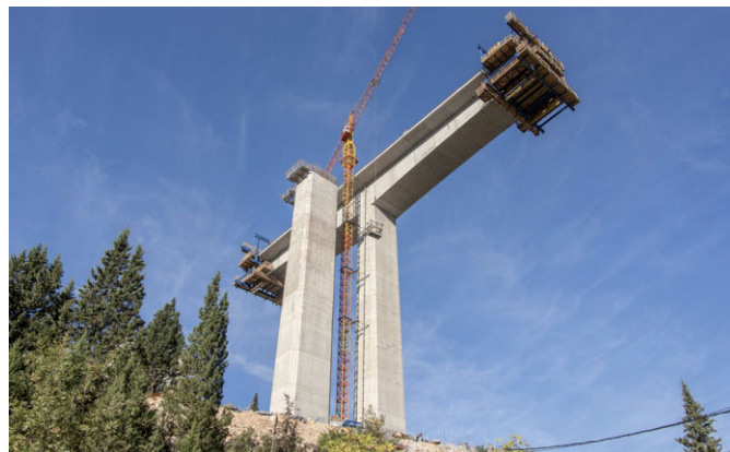
Fig. 3. The total number of ten Doka-Cantilever forming travellers were placed into their correct starting positions with the help of gantry crane parts. (© Doka)
