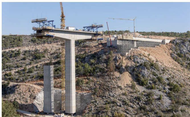
Fig. 1. High-performing at lofty heights: Ten Doka-Cantilever forming travellers allow for rapid and safe construction of both bridges along the Corridor Vc.
