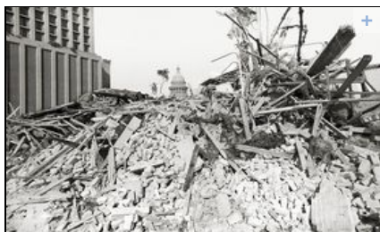
Demolition of Charles B. Cook Funeral Home, 1100 Colorado St., looking northeast in 1983. The 26-story Westgate Tower is on the ... Read More
